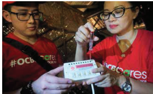
Volunteer dari Bank turut membangun fasilitas penerangan dan perbaikan sekolah. The Bank’s volunteers helped to build lighting facilities and repair schools.
